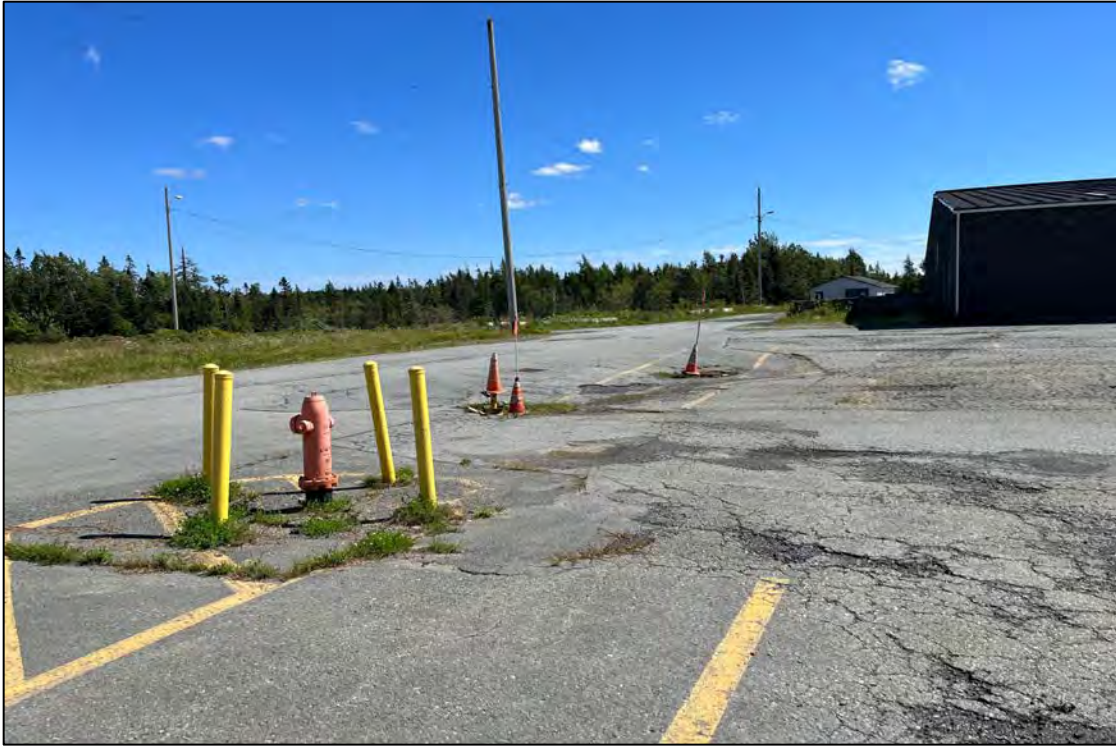
Plate 18: A fire hydrant, power poles, and eroding manholes/storm drains, looking south.
