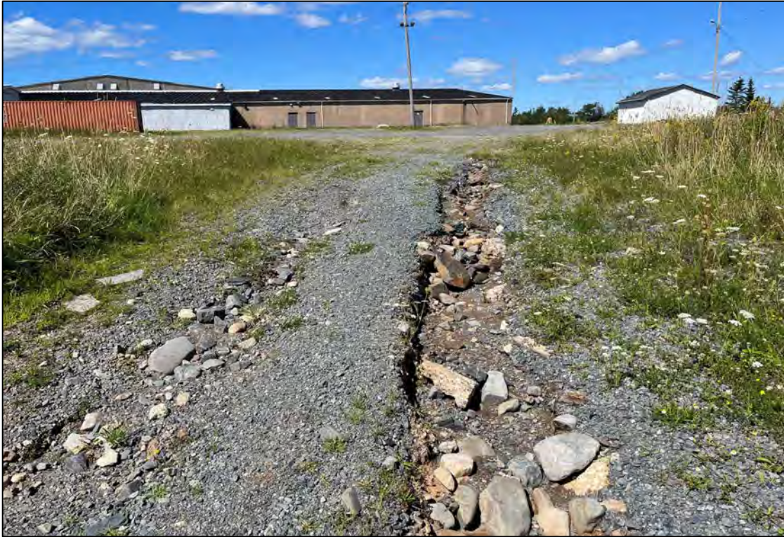
Plate 27: A gravel road leading from the gravel driveway at the south end (back) of the Halifax Exhibition complex. Note the large rock and concrete fill visible under the eroding gravel, looking north.
